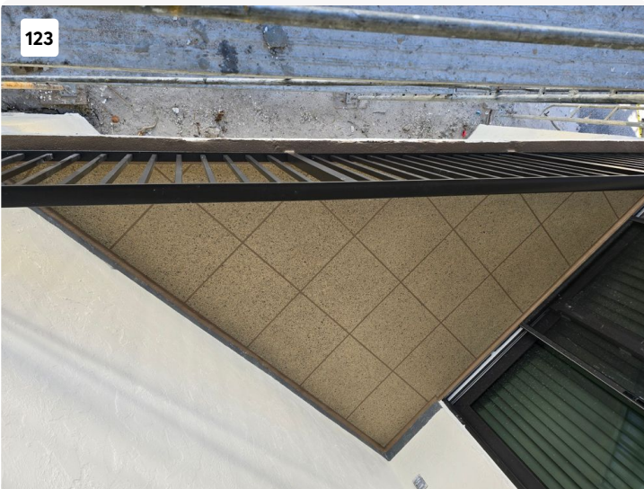
Rear balcony with new railings and polyurethane water-proofing membrane with gemstone acrylic coating.
