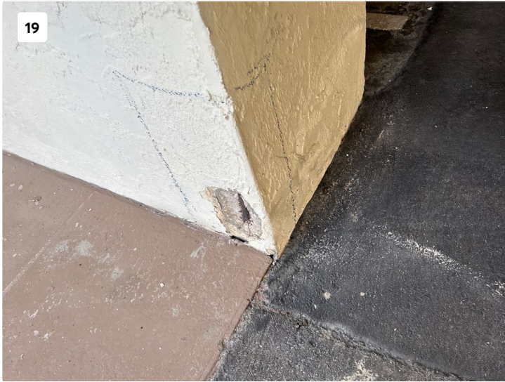
Garage column spall.
