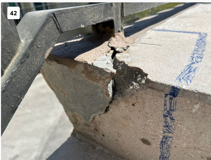
Failed post pocket and existing railing.
