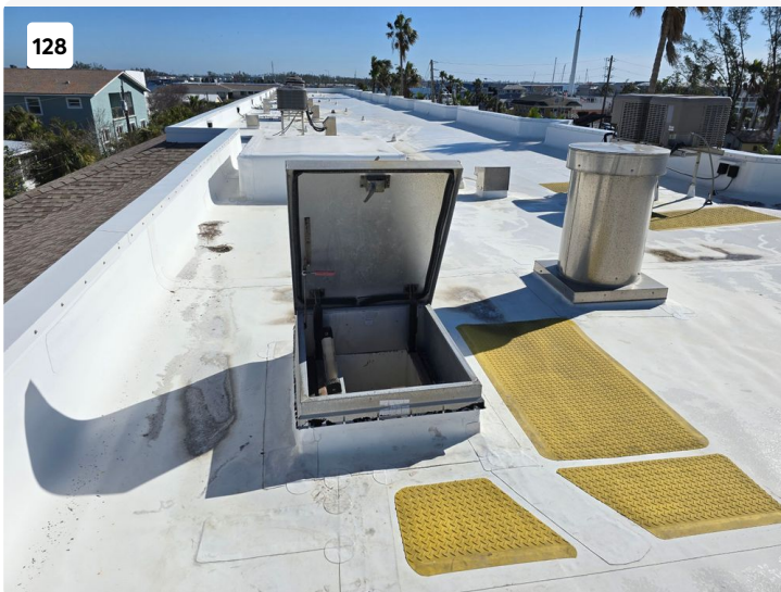
TPO flat roof installed circa 2022.
