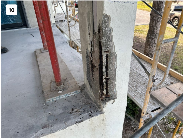
Vertical spall in balcony column.
