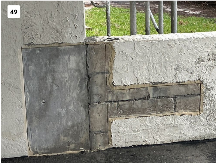
Delaminated stucco removed at intersection of CIP column and CMU block knee wall.
