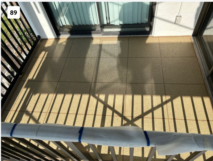
Rear balcony with new railings and polyurethane waterproofing membrane with gemstone acrylic coating.
