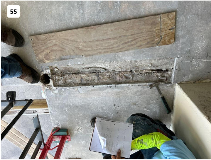
Cracking through topping slab at intersection of hollow cor panels on walkway.
