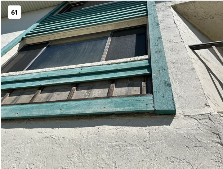
Damaged and rotting wood trim to be removed and replaced. Exposed CMU block underneath to be water-proofed.
