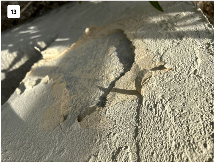
Areas of deteriorated stucco in exterior garage walls.
