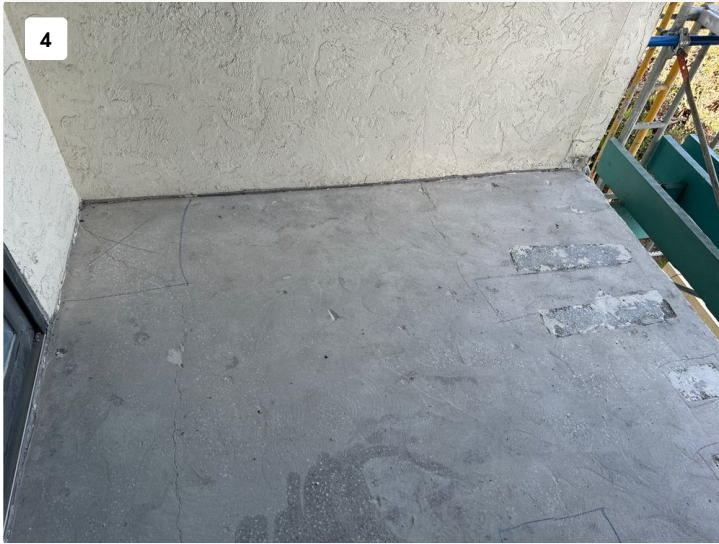
Sounding and marking of balcony deck spalls.
