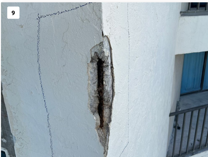
Vertical spall in corner column.
