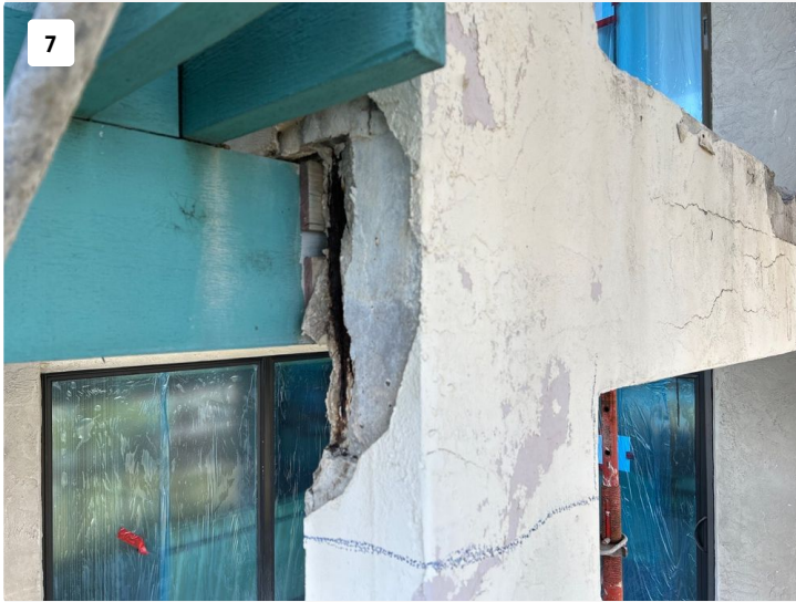
Spall in balcony column behind wood outrigger structure. horizontal spall at edge of balcony.
