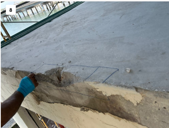
Slab edge spall on balcony.
