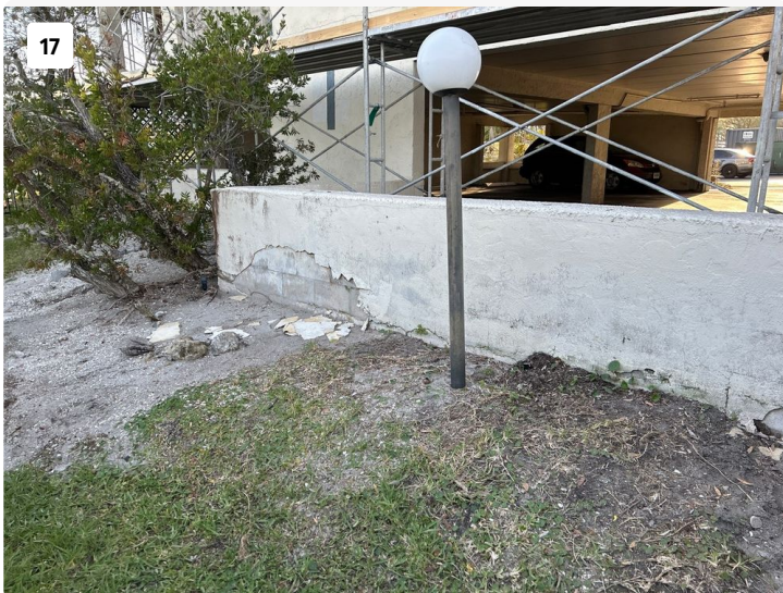
Failed stucco on exterior garage wall.
