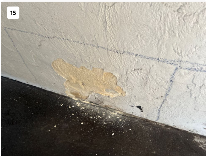
Area of deteriorated stucco in interior garage walls.
