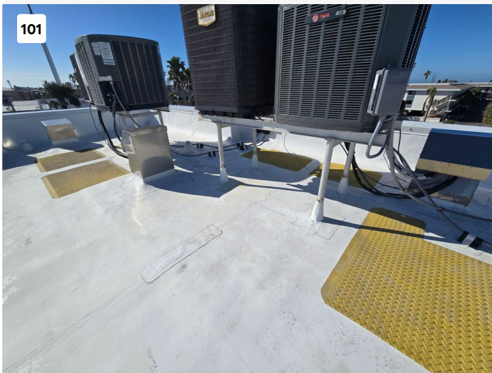
Mechanical units elevated on stands.
