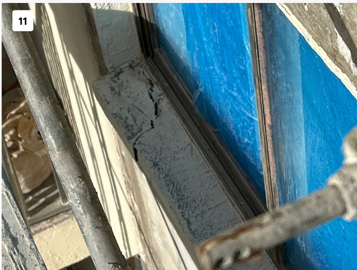
Spall in window sill.
