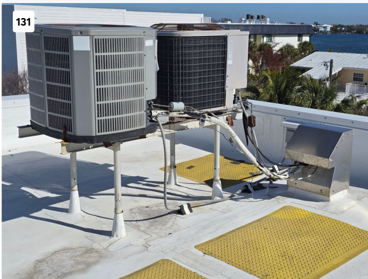
Mechanical units elevated on stands.
