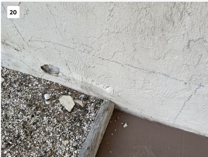
Area of delaminated stucco.
