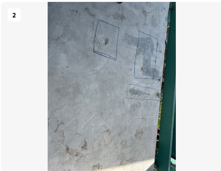
Sounding and marking of balcony deck spalls. Previous repairs visible.
