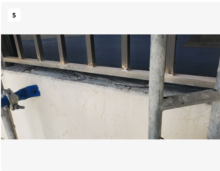
Cracking in balcony coating.
