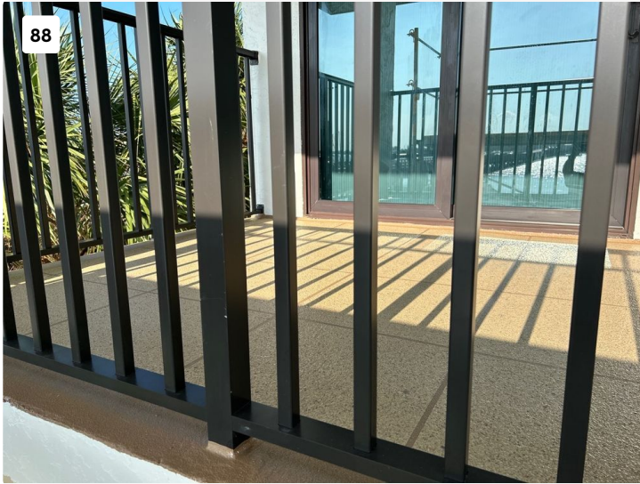
Rear balcony with new railings and polyurethane waterproofing membrane with gemstone acrylic coating.
