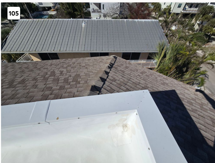
Shingles damaged during recent hurricane event.
