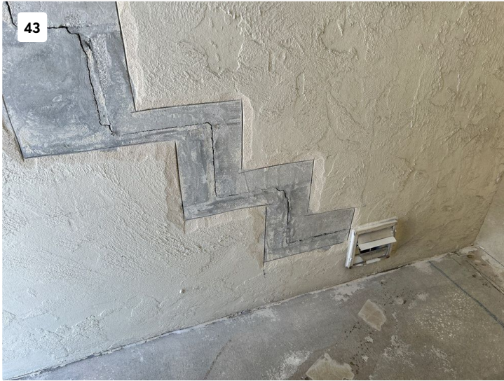
Stucco repair around stair step crack.
