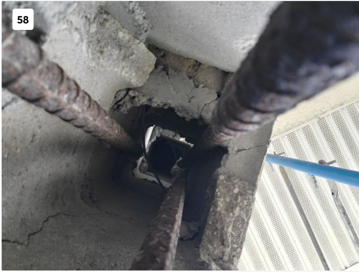
Cell with rebar that was never filled with concrete.
