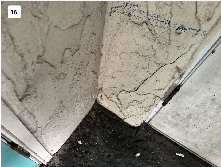
Vertical spall adjacent to garage door.
