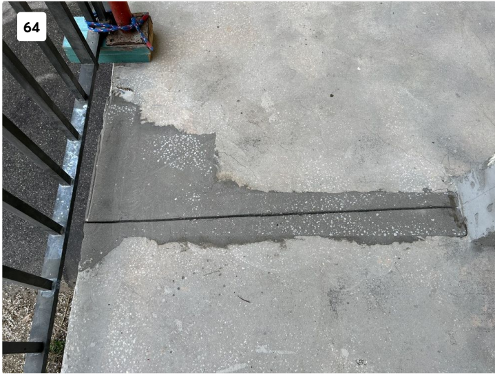
Joint created at location of walkway cracking.
