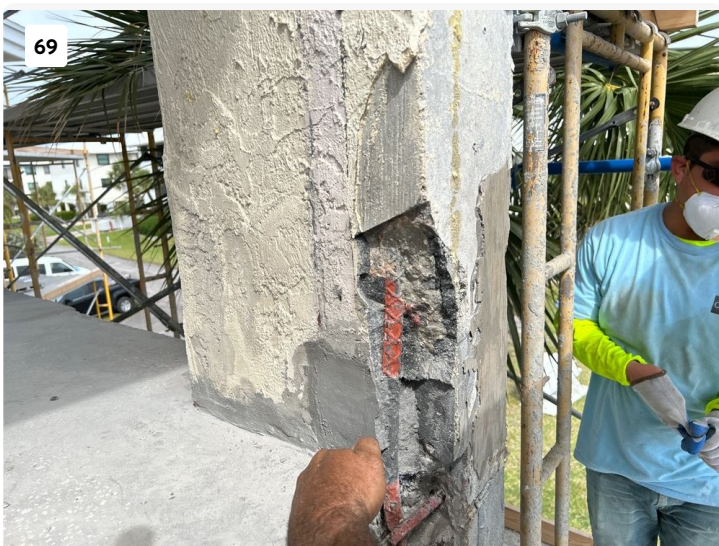
Failed previous concrete repair in balcony column.
