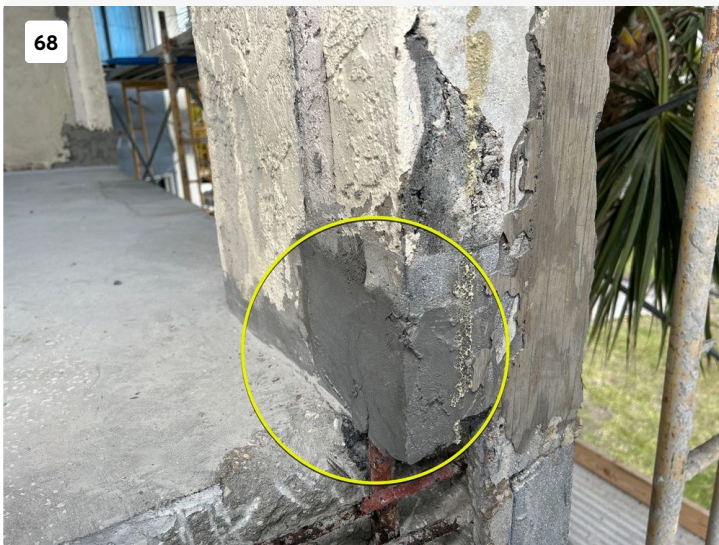
Failed previous concrete repair in balcony column.
