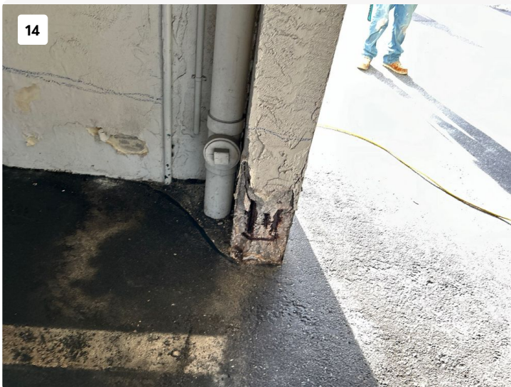
Garage column spall.
