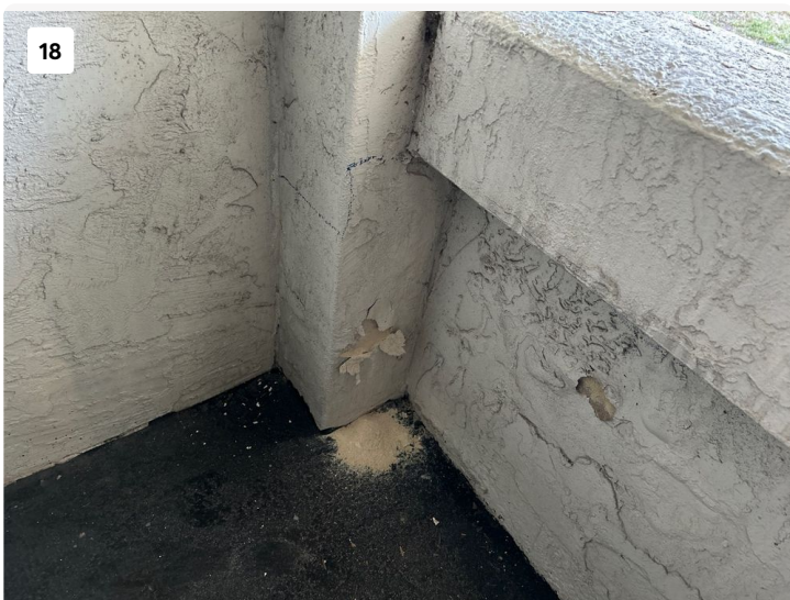
Areas of deteriorated stucco in interior garage walls.
