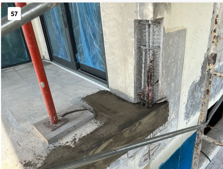
Completed balcony slab edge concrete repair and in progress vertical concrete repair.
