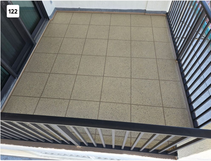
Rear balcony with new railings and polyurethane water-proofing membrane with gemstone acrylic coating.
