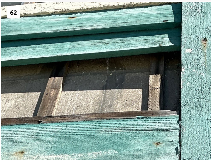
Damaged and rotting wood trim to be removed and replaced. Exposed CMU block underneath to be water-proofed.
